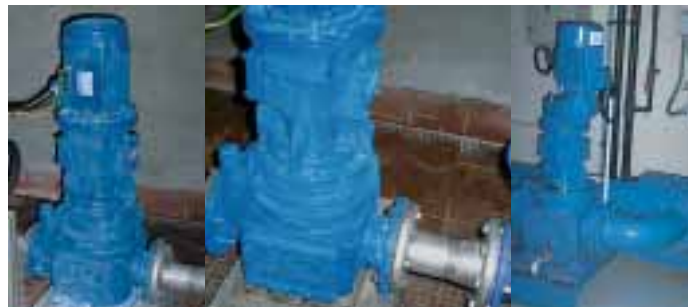
Sludge recycling: Porto-Freixo and Versailles-Sevesc
